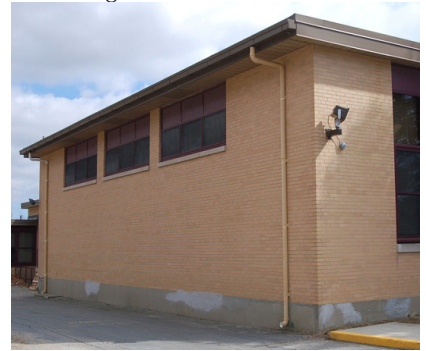
previously repaired areas at concrete foundation, 1959 building
