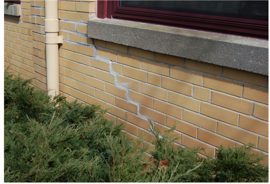
Step cracking below window sill, west elevation original building
