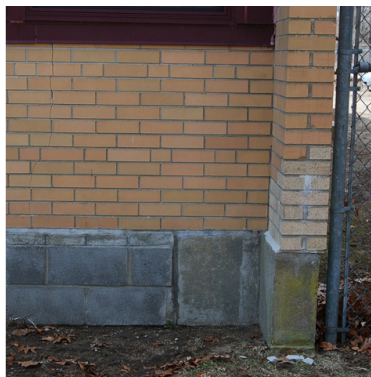
Displaced brick at northeast corner of 1959 classroom wing
