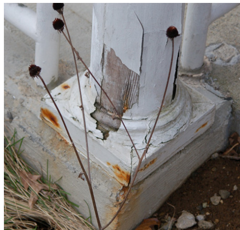
Wood rot and peeling paint at base of entry post.
