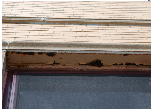
Rusted lintel at auditorium
