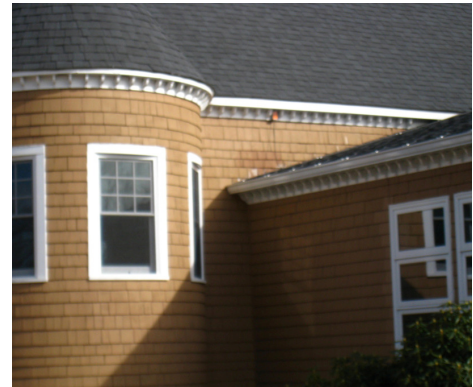
peeling paint at junction between building wall and roof, west elevation
