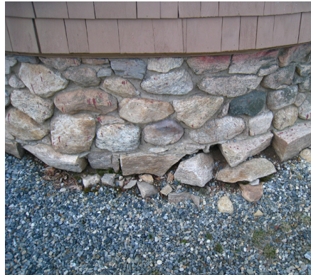
Loose foundation stones at north elevation
