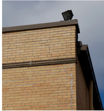
Cracked and sealed brick at southeast corner of auditorium
