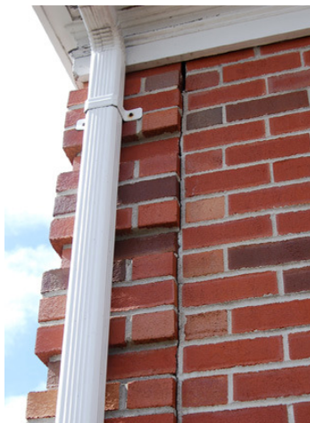
Northeast corner crack.
